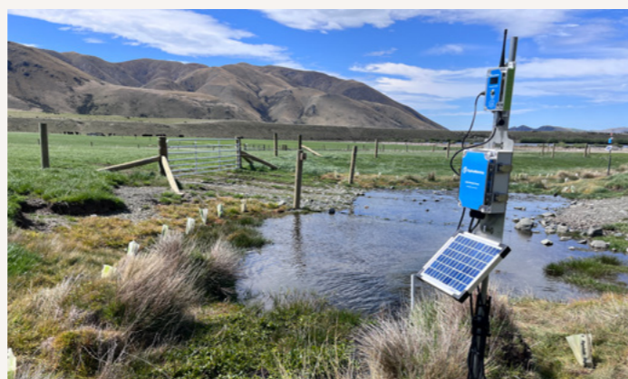
HydroMetrics groundwater monitoring system
